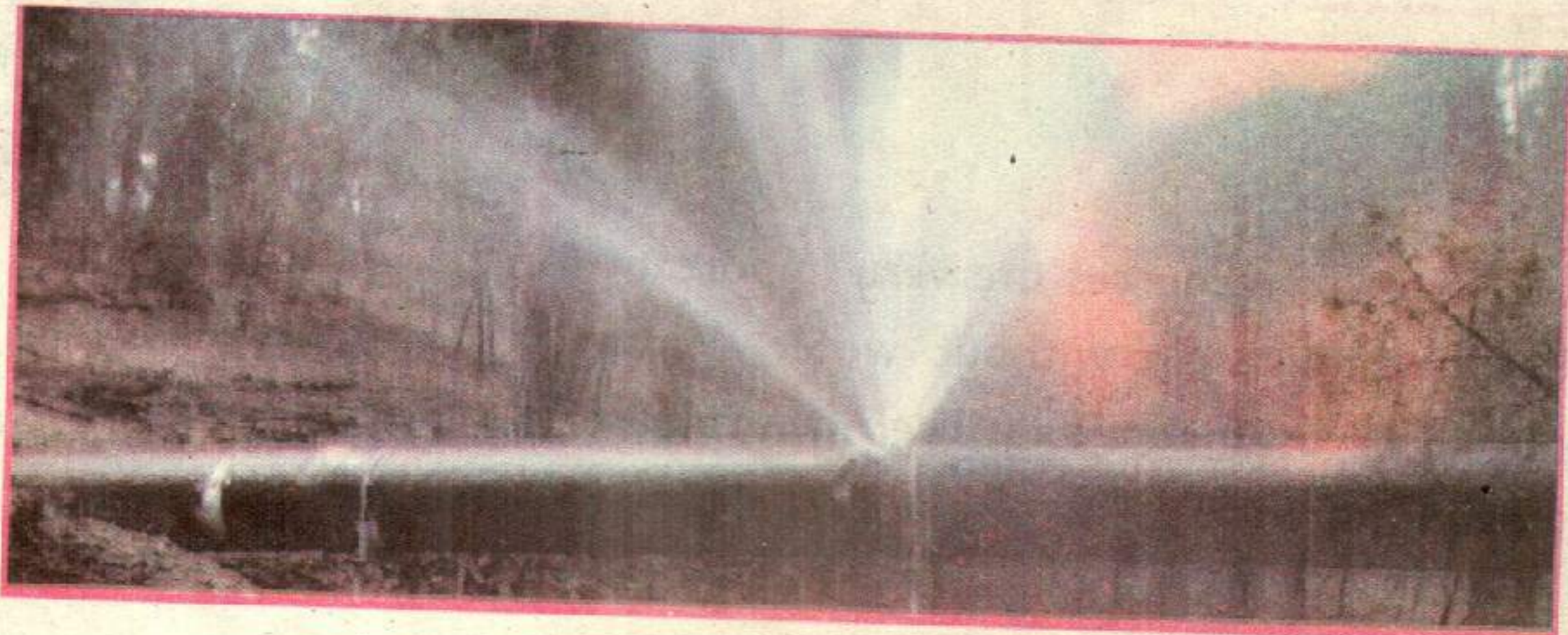
Leakage of pipeline
